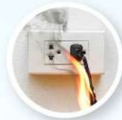
Lightning- induced power surge?
